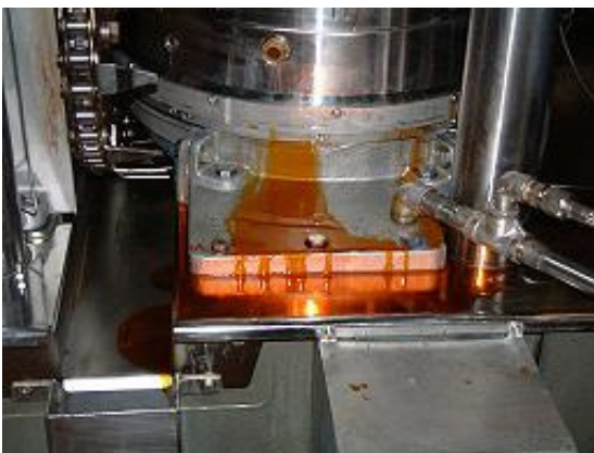
Angelus can seamer oil leakage found after using red dye
